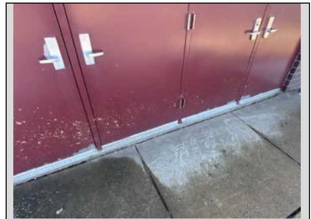
Hollow metal doors – paint peeling at the bottom.
