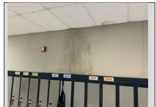
Staining on acoustic wall panel
