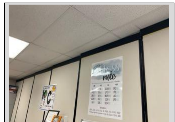
Operable partition not aligning.
