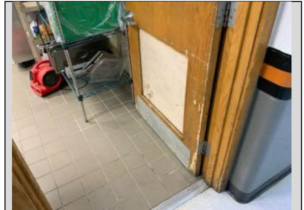
Worn wood door with wood door frame.
