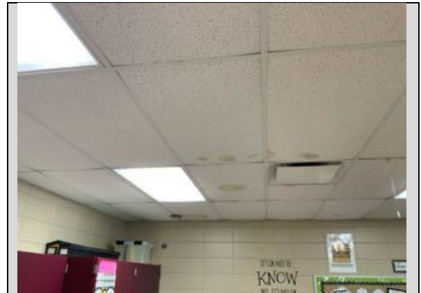
Typical water damage and sagging of acoustical tiles.
