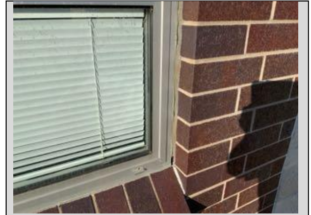
Typical sealant joint failure at windows
