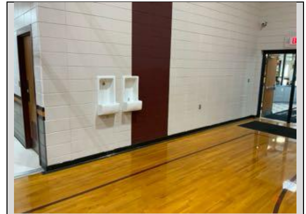
Non-accessible drinking fountains.
