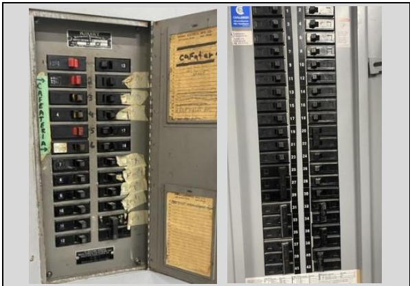
Various aged electrical panels
